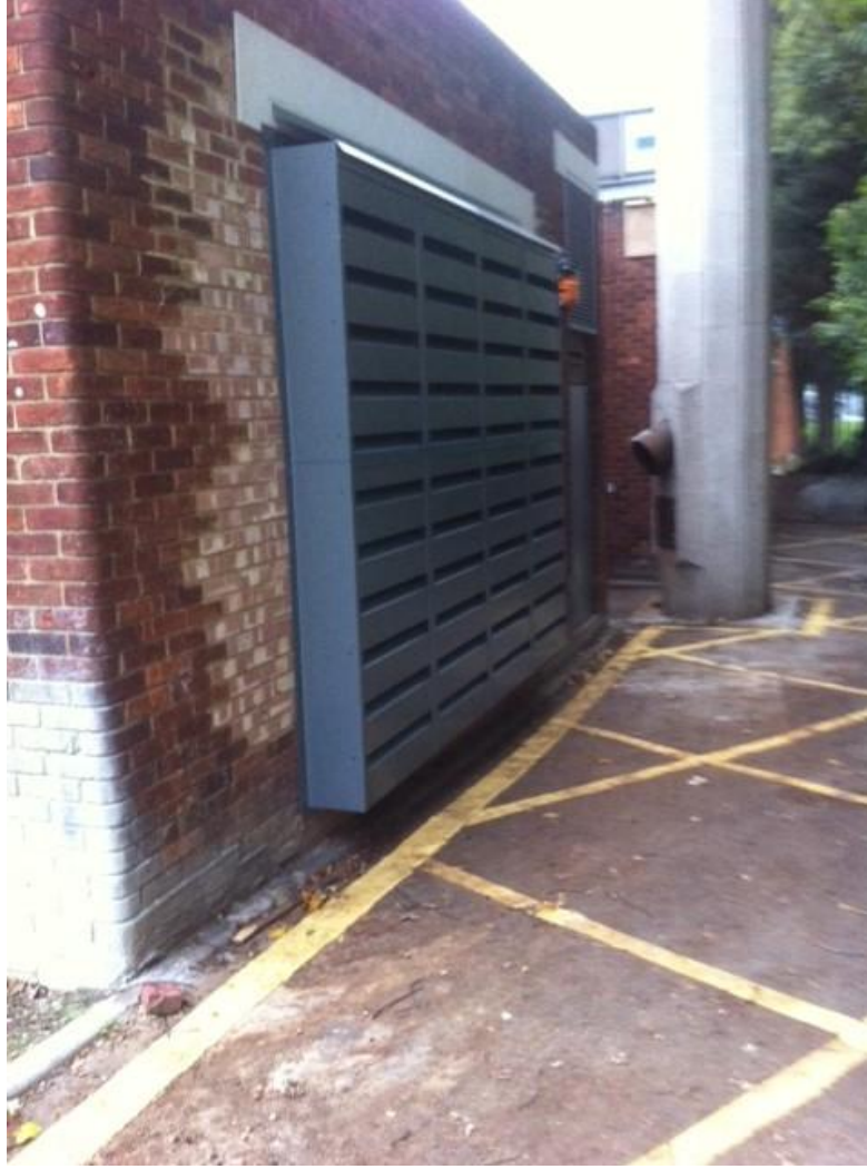
Acoustic louvre to back of plant room
